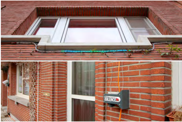
Figure 4: Shush . Top: LEDs on second floor. Bottom: control unit next to front door. Engraving reads, “Enjoy the silence”.
